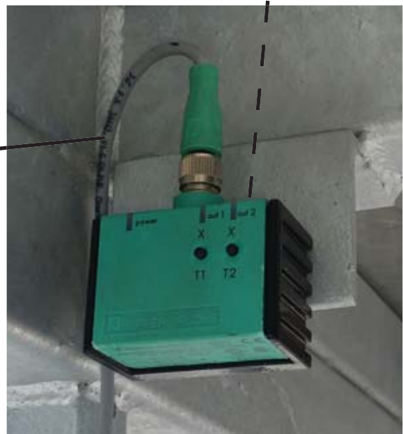
INCLINOMETER ON BRIDGE
