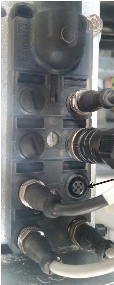
JUNCTION BOX NEAR CYLINDER
