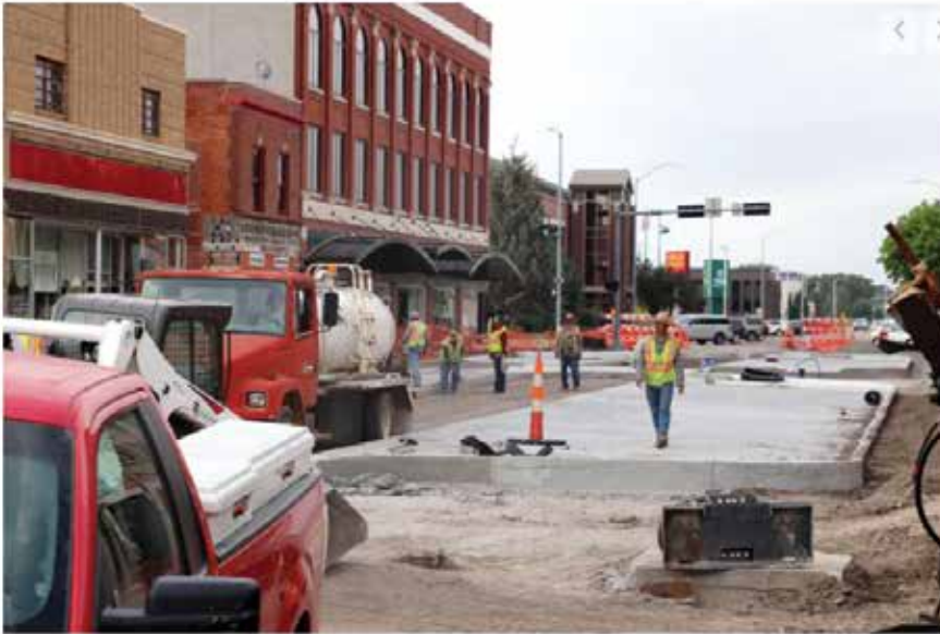
A Paulsen Inc. worker walks north Friday morning on one of the recently laid concrete parking strips on North Platte's North Dewey Street between Fourth and Fifth streets. Behind him, four colleagues continue laying sand where Dewey's 1916 paving bricks will soon be reset atop a 6-inch-deep concrete base that has yet to be poured between the parking strips.
