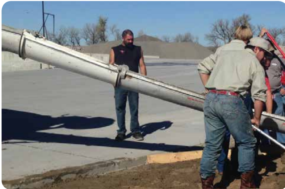
Mid Plains Community College Decorative Concrete Seminar put on by our Ready-Mix division at the North Platte Paulsen Inc. plant.
