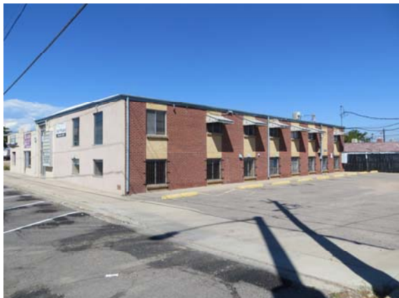
Figure V-3. Stucco was applied to the south wall of the Derby Professional Building at 6401-6405 E. 72 nd Avenue (5AM3132). The east wall retains its original character-defining features from its construction in 1949.
