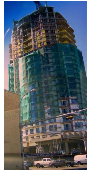
Condominium tower under construction in downtown Edmonton. Sustained leadership and vision for downtown have created the conditions for a dramatic increase in the downtown population.
