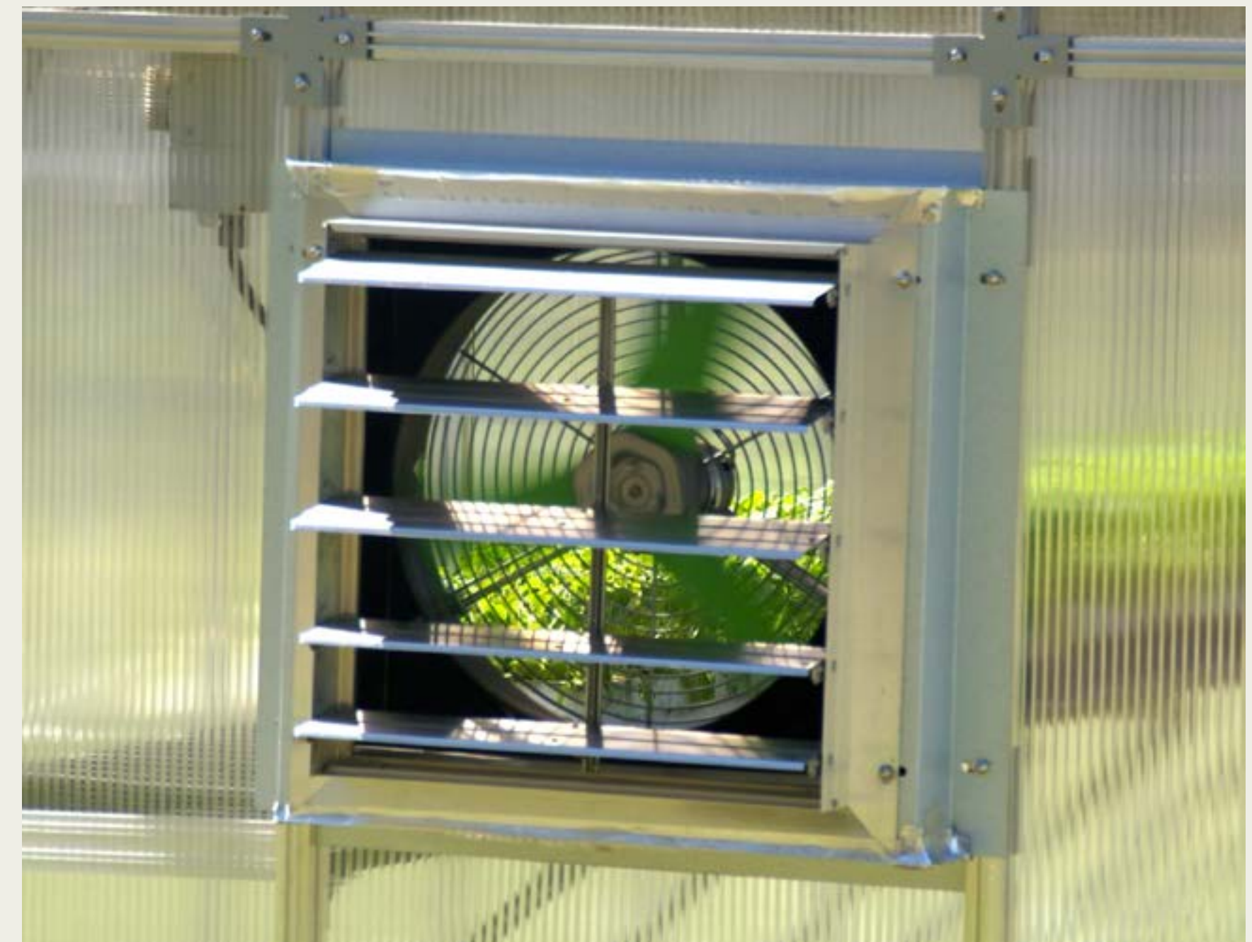
A Powered Ventilation System (PVS) with exhaust fan keeps a greenhouse 10 degrees cooler than traditional ridge vents.
