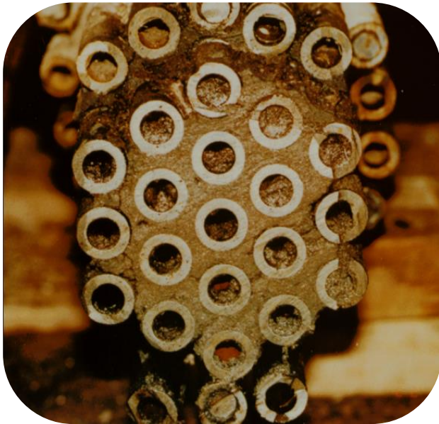
Fouling in heat exchangers ( http://scopewe.com )
