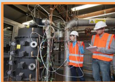
250kW PF coal & biomass air/oxyfuel test facility
