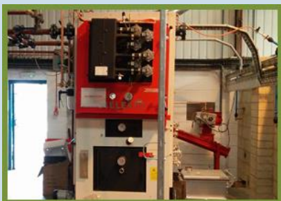
240kW biomass chip/pellet grate boiler
