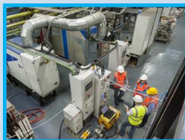
300kW CHP gas turbines
