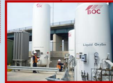
Gas mixing facilities: synthetic /modulated flue/process gas
