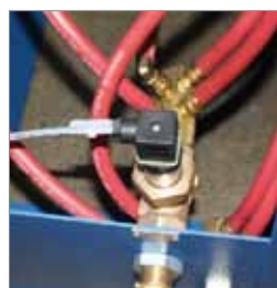
FLOW CONTROL INSTRUMENT (water control switch) installed in water feed
