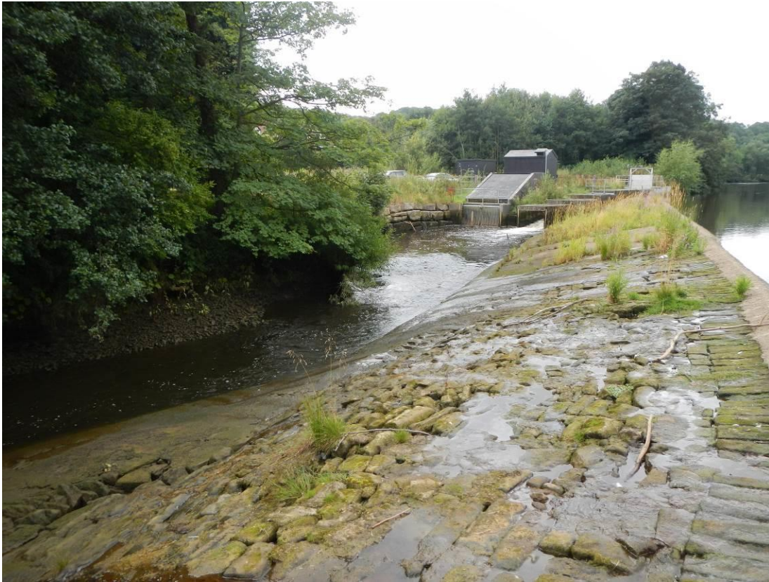
Figure 8. The size of the weir structure and concrete ridge along its crest also render it a significant obstacle to eel migration.
