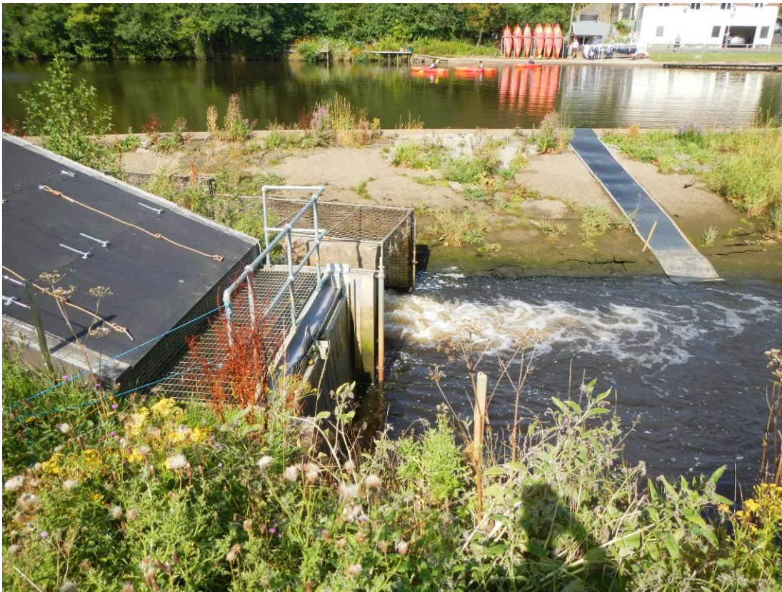
Figure 7. The d/s end of the fish pass, the level of which already appeared very close to the d/s water level. Ideally, a Larinier pass should terminate well below the d/s water level to allow fish to enter the plume within the water column of the pool.
