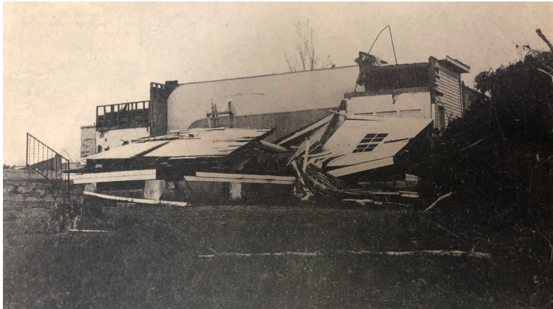
... And, this is all that is left of the structure which was in the path of the violent tornado funnel which swept with destructive force through Robertson County last week. The church will be rebuilt.
