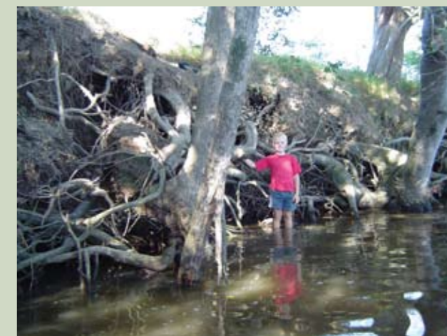
A section of riverbank undercut to 2 m. Not even the tree roots were able to hold the soil together.
