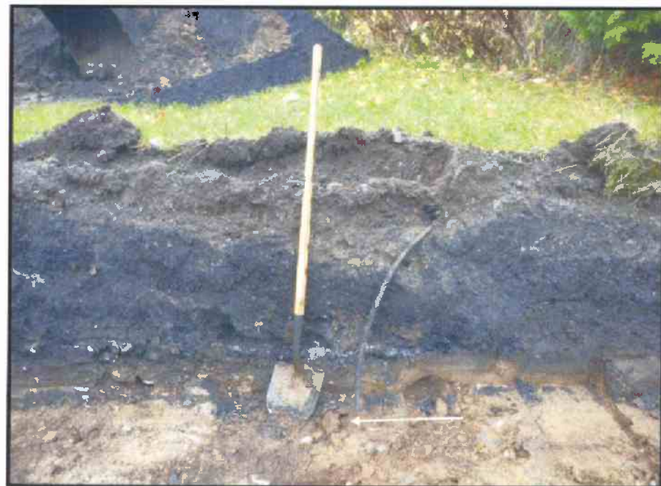
Image 88: Electrical Conduit Associated with Asphalt in Grid 5 Western Anomaly Investigation Area (looking southwest)
