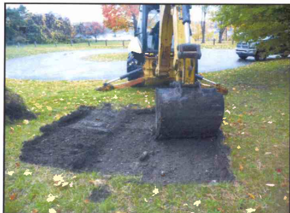
Image 64: Topsoil Stripping of GPR Anomaly in Grid 5, South of Paved Laneway and Turnaround (looking north)
