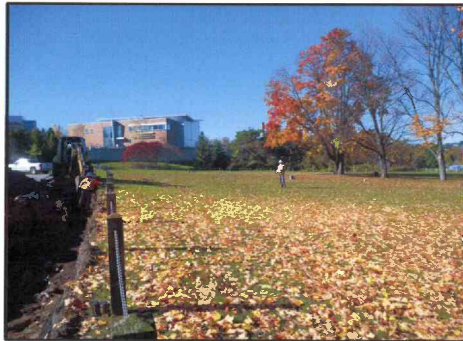
Image 61: Topsoil Stripping of South Cemetery Boundary and Recording Elevation Points with Topcon (looking west)
