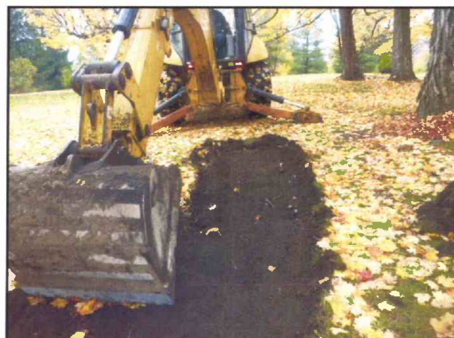
Image 65: Topsoil Stripping of GPR Anomalies in Grid 3 East of Cemetery (looking southeast)
