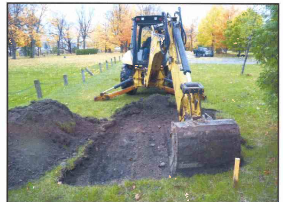
Image 63: Topsoil Stripping of GPR Anomaly on West Side of Grid 5 (looking east) * note stake represents mapping datum
