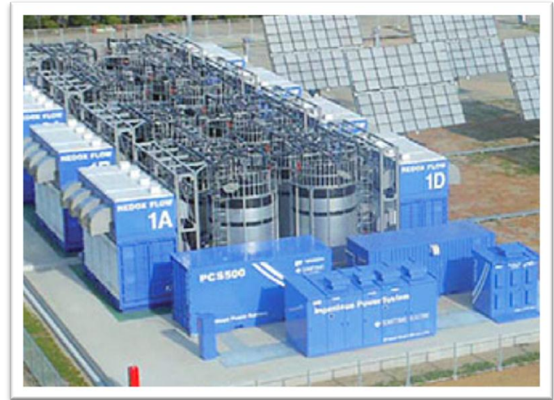
STORAGE: Sumitomo Electric Redox Flow Battery
