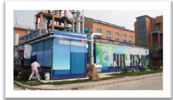
2 MW PEM Fuel Cell Plant
