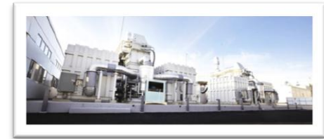
59 MW Gyeonggi Green Energy facility Hwasung City, South Korea.
