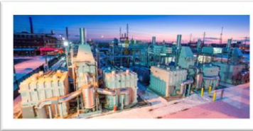
3.7 MW DMC Fuel Cell Modules
