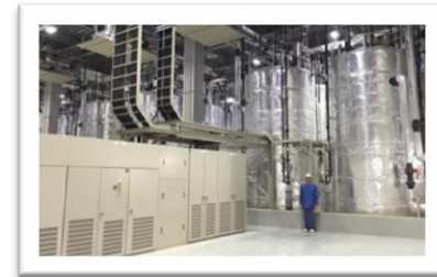
An electrolyte tank in the building that stores the storage battery (source: HEPCO)
