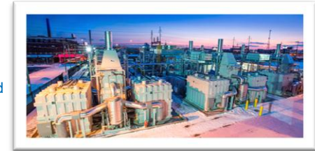
15 MW Dominion Bridgeport Fuel Cell Plant, Bridgeport, Connecticut, U.S.A., uses 0.6 of a Ha. of land and powers approximately 2% of Connecticut Renewable Portfolio Standard.
