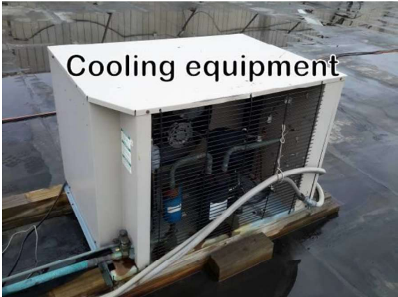
Standing water on roof
