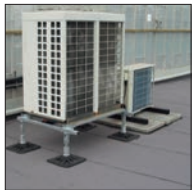
Plant & Equipment Support System.
