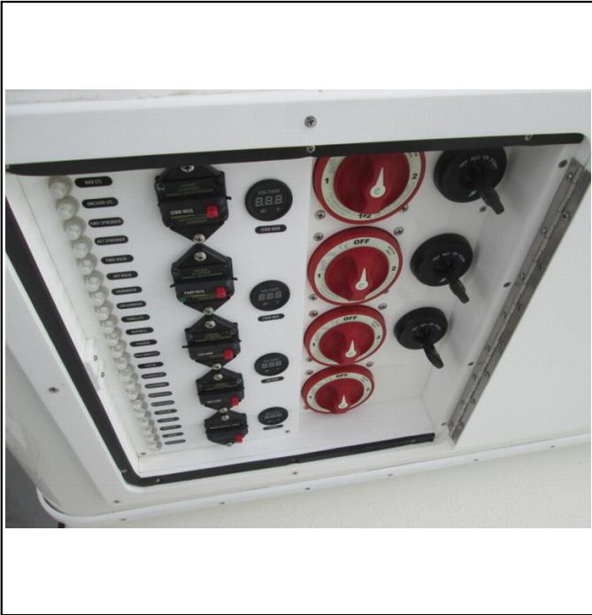
Battery management panel, photo 34.
