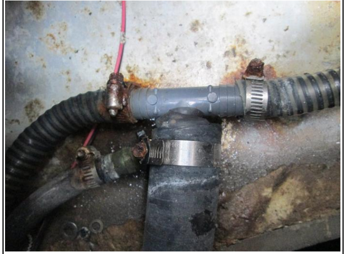
Plumbing under aft cockpit deck at aft facing seat, photo 43.
